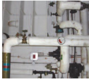
Asbestos insulation on pipes
